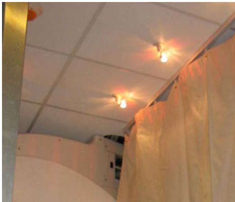
Magnet Room Lighting
