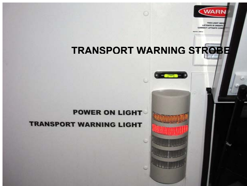
Figure 60: Lift Transport Warning Strobe
