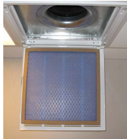
Downstream Blower Filter Access
