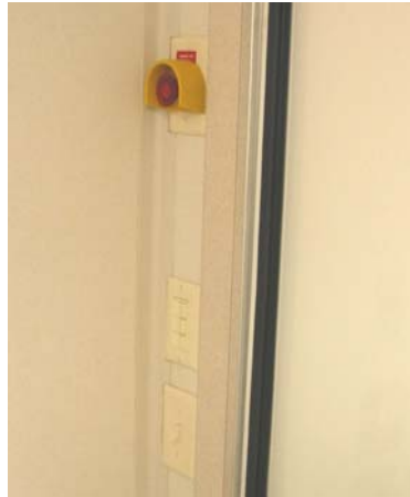
Control Room Lighting and E-Stop
