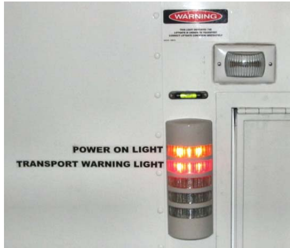
AC Power Warning Light and Transport Warning Light Figure 59: Warning Lights
