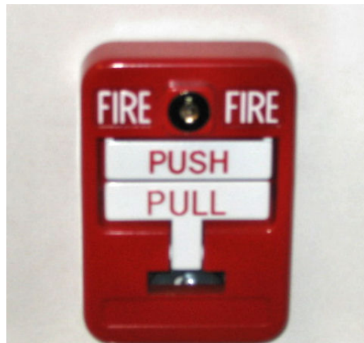
Figure 27: Fire Alarm Pull Station
