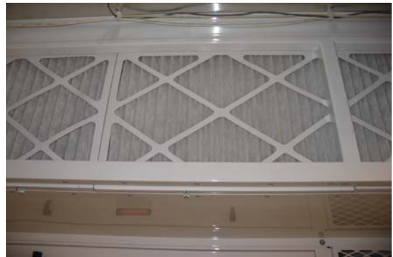
HVAC Filter Access
