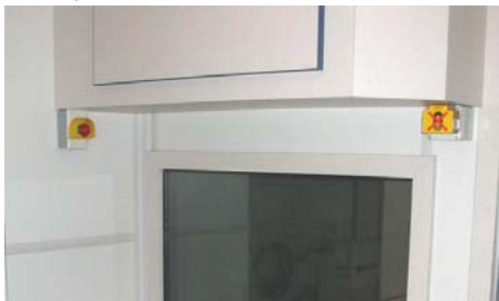
Scan Room E-Stop and Magnet Quench Controls
