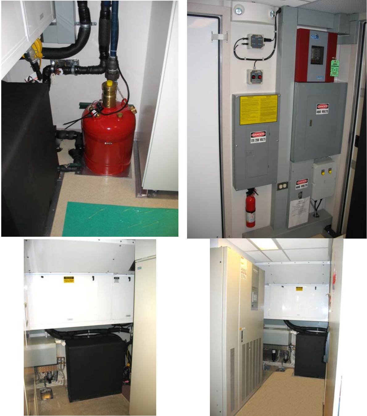
Figure 6: Equipment Room Overall
