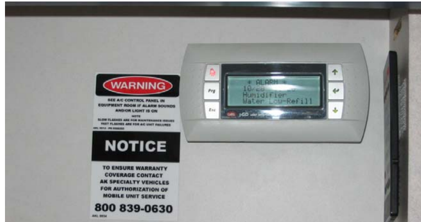
Figure 41: A/C / Chiller Alarm Panel
