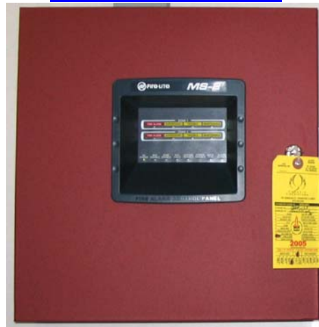
Figure 26: Fire Alarm Control Panel
