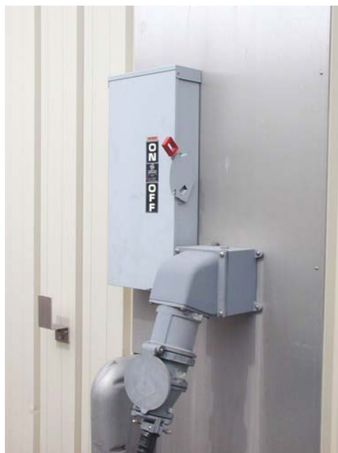
Figure 35: Shore Power Connection
