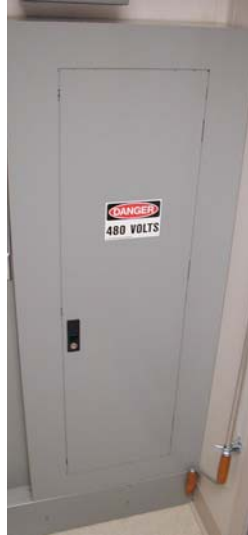
Figure 34: 480V AC Electrical Panel
