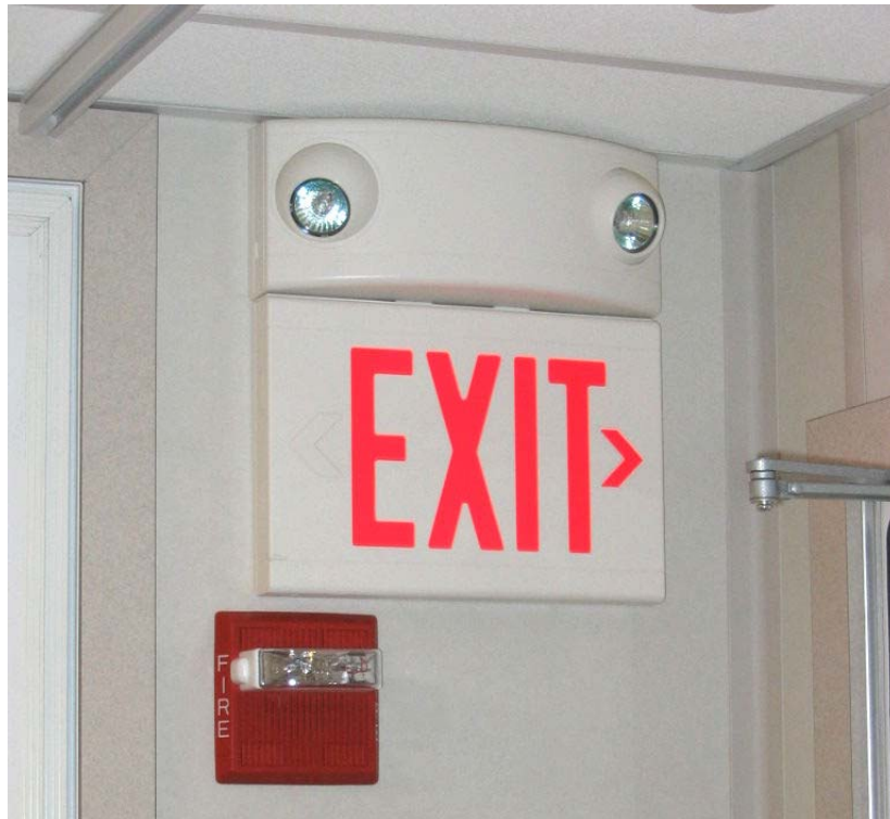
Figure 51: Emergency Dual Beam Lighting
