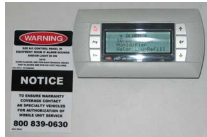
Air Conditioning Trouble Light & Alarm
