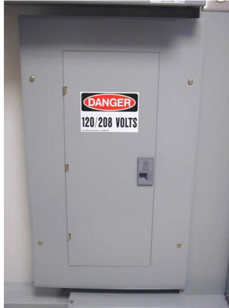
Figure 33: 120/208V AC Electrical Panel
