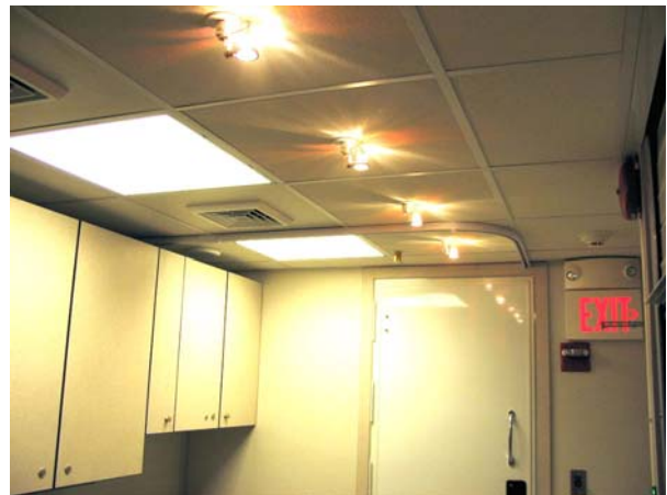
Figure 56: Control Room Lighting
