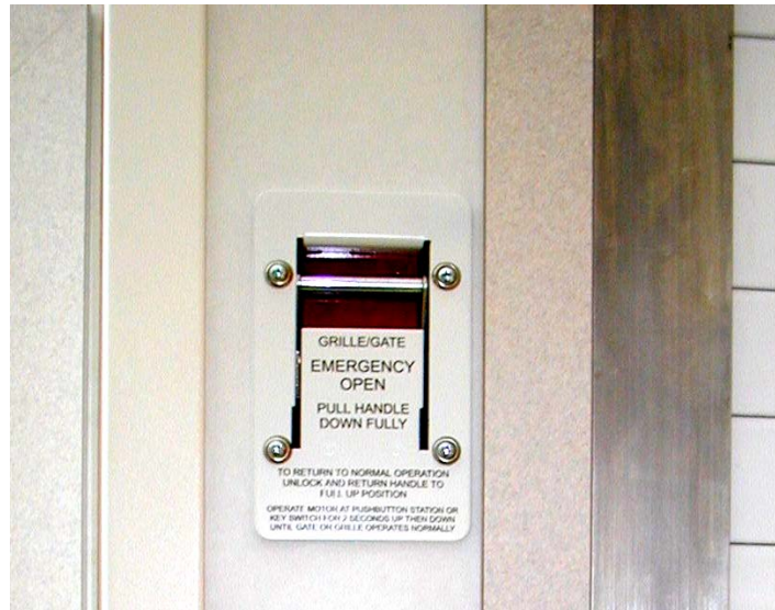
Figure 31: Roll Door Emergency Release
