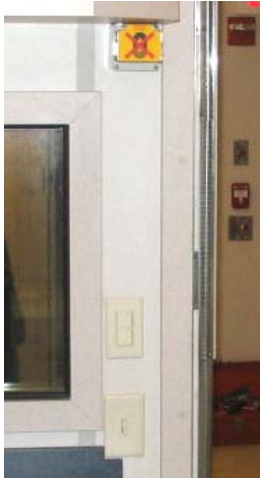
Scan Room Lighting and Magnet Quench Controls
