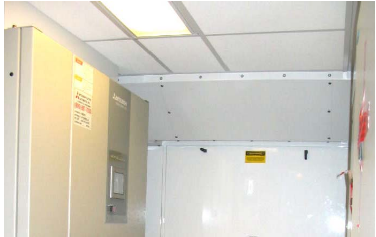
Figure 55: Equipment Room Lighting
