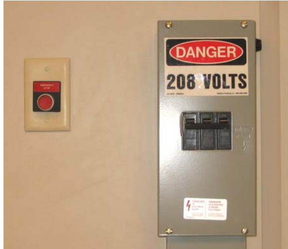
Figure 17: Emergency Shutdown Buttons
