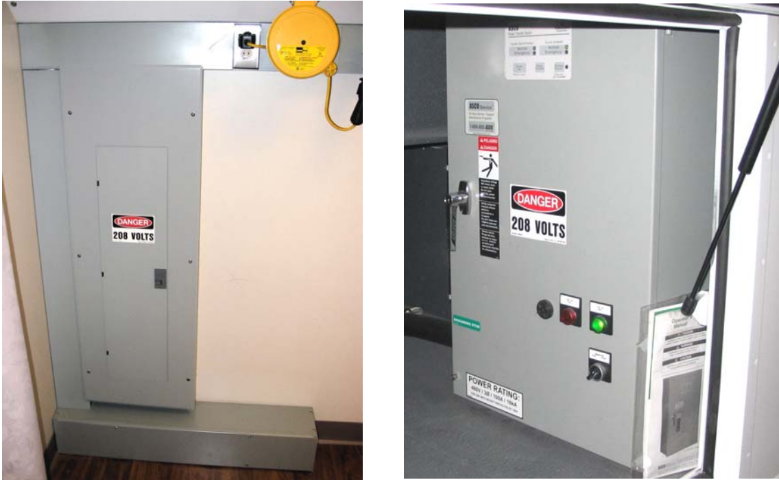
Figure 20: 120/208V AC Electrical Panel and ATS
