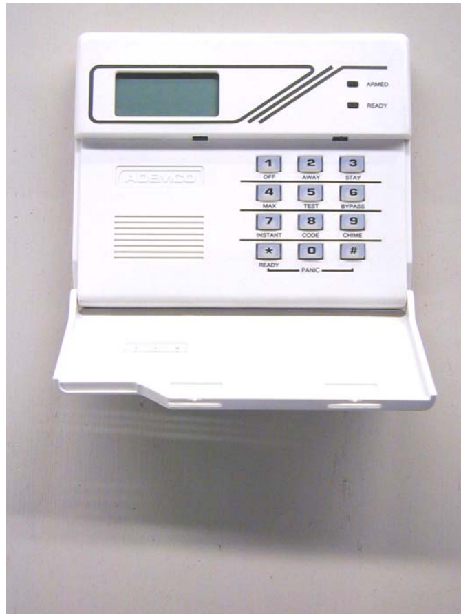
Figure 28: Intrusion Alarm Keypad
