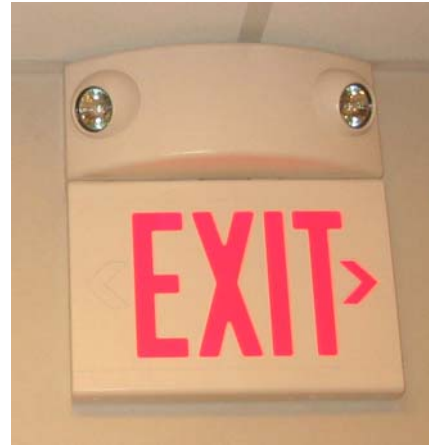
Reception Area Emergency Light
