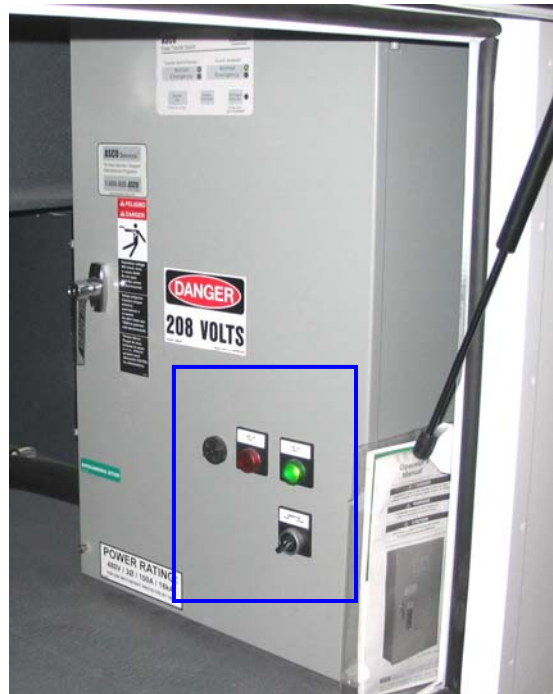
Figure 21: 208V AC Phase Power Monitor on ATS
