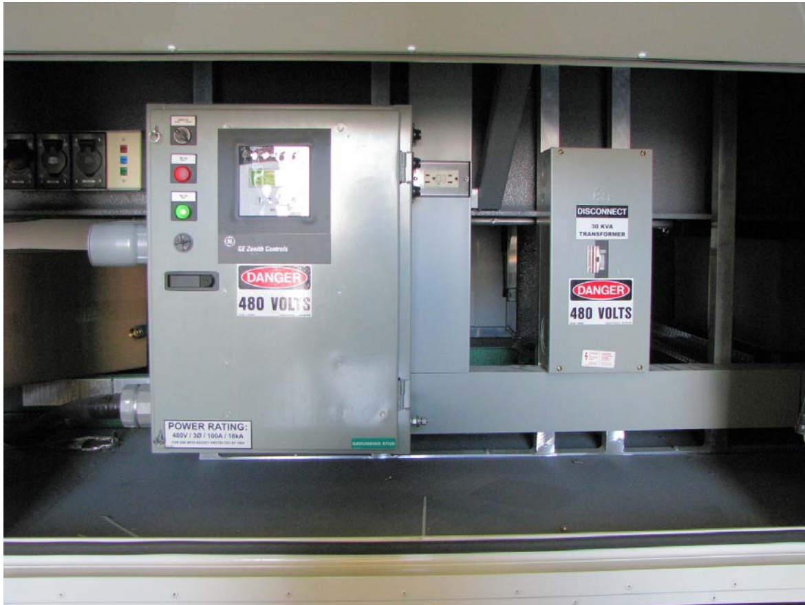
Figure 26: Automatic Transfer Switch and Phase Power Monitor
