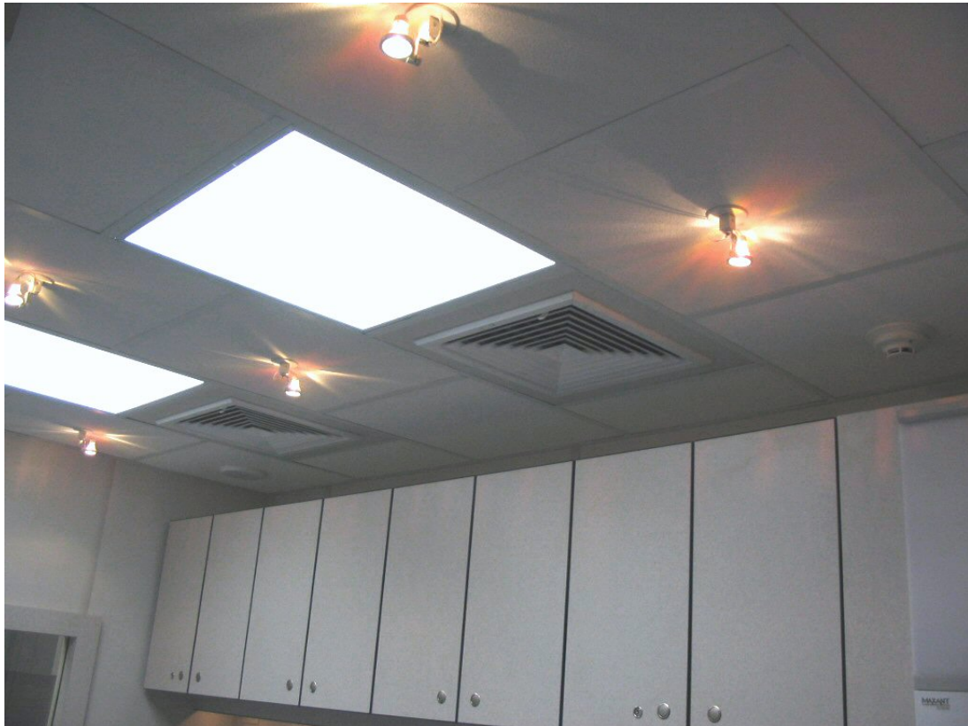
Figure 52: Control Room Overall Lighting
