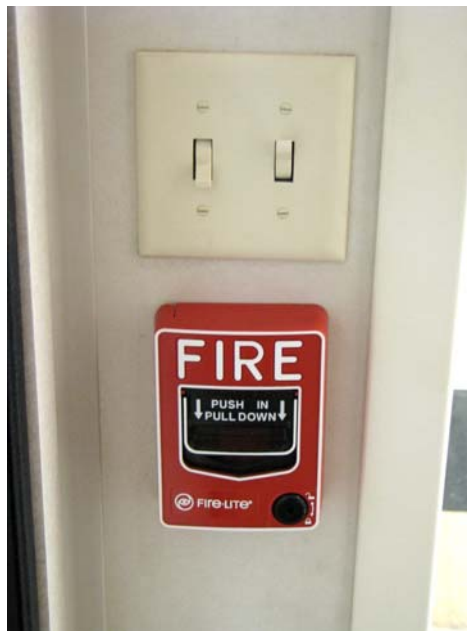
Figure 20: Fire Alarm Pull Station
