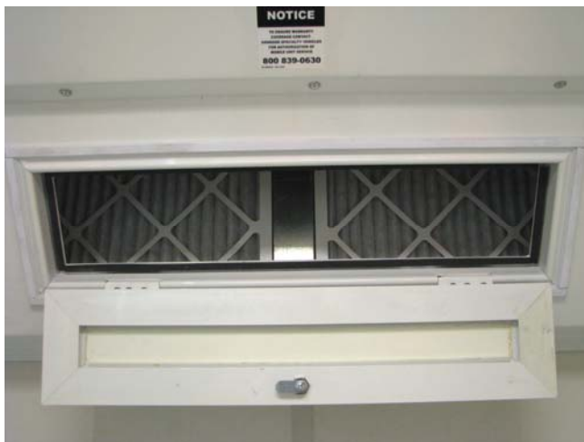
HVAC Filter Access
