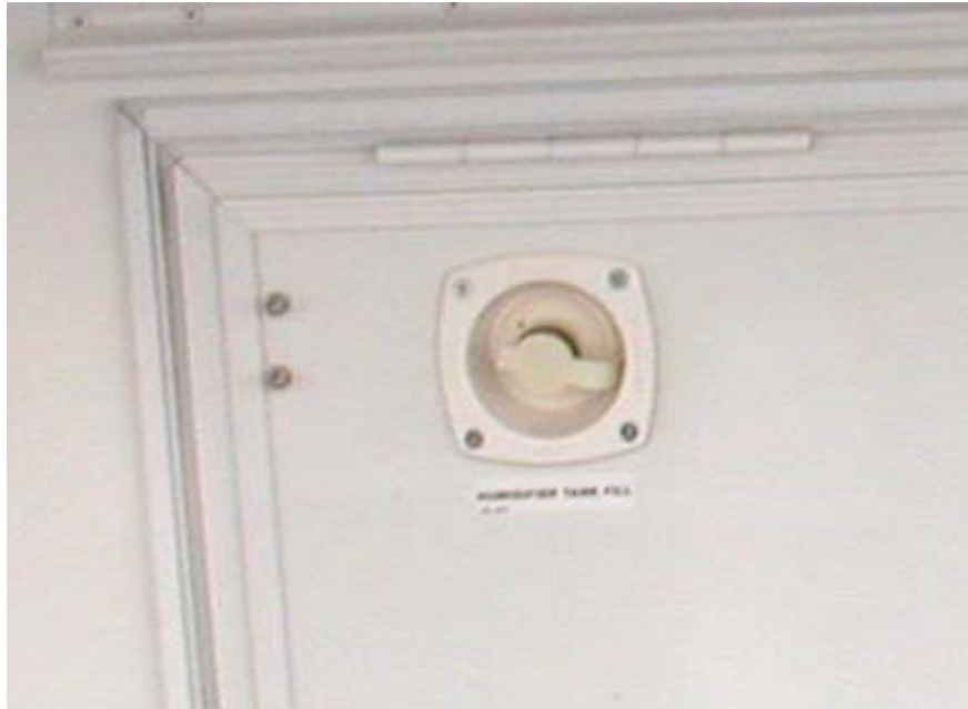
Figure 27: Humidifier Tank Fill
