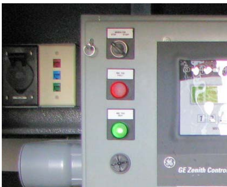
Figure 30: 480V AC Phase Power Monitor
