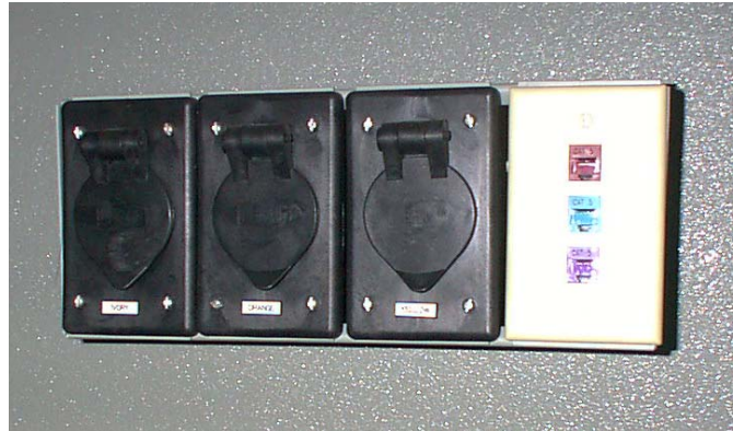
Figure 12: Phone & Data Line Connections
