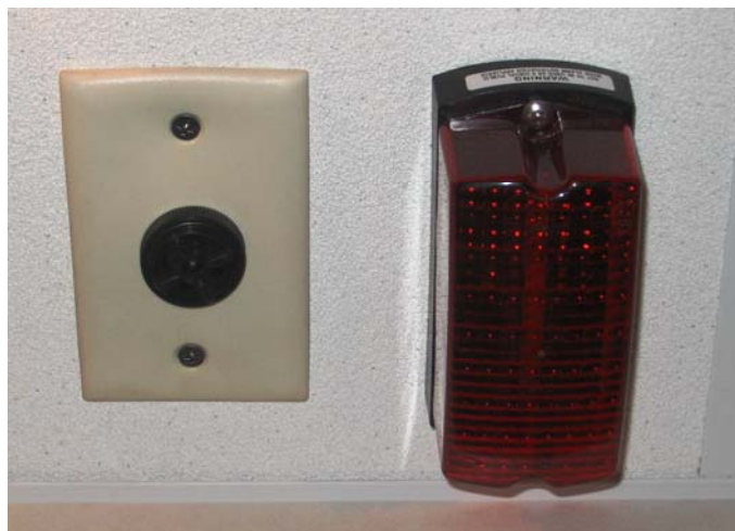
Figure 42: Platform Lift Strobe & Alarm
