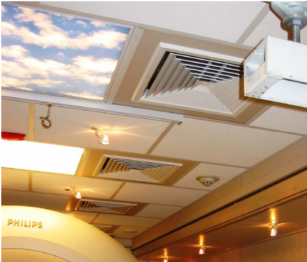
Figure 53: Gantry Room Overall Lighting
