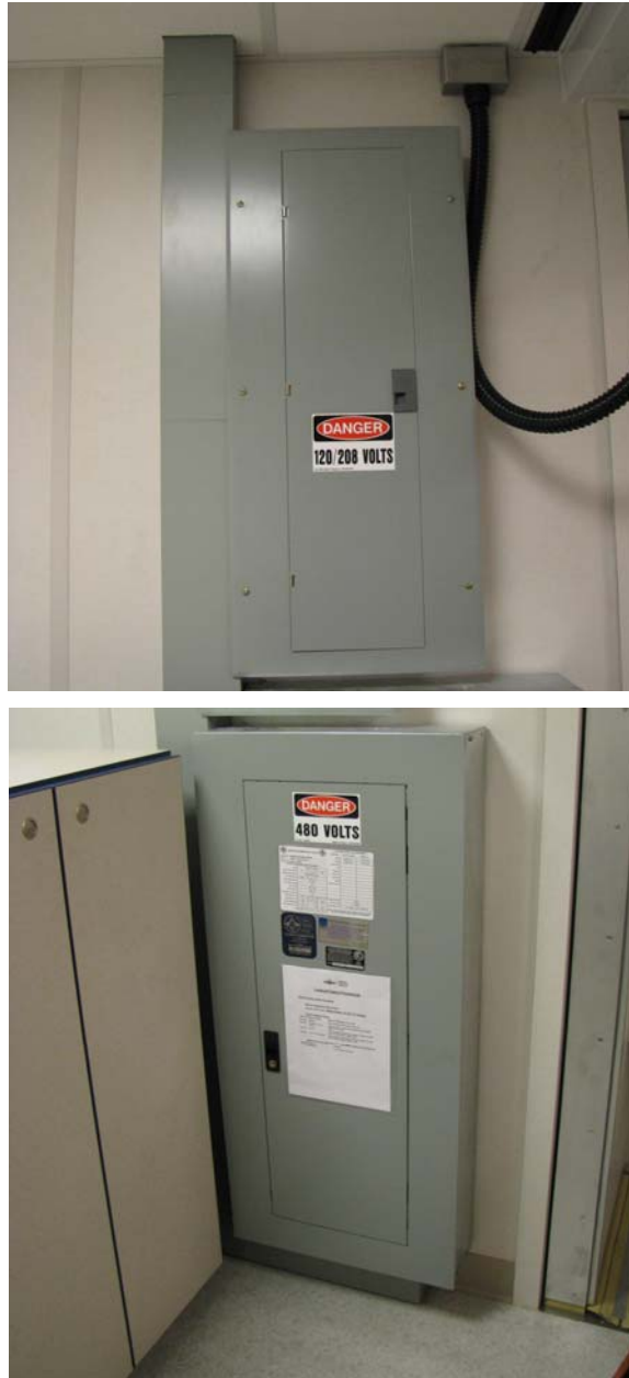
Figure 28: 480V and 120/208V AC Electrical Panels
