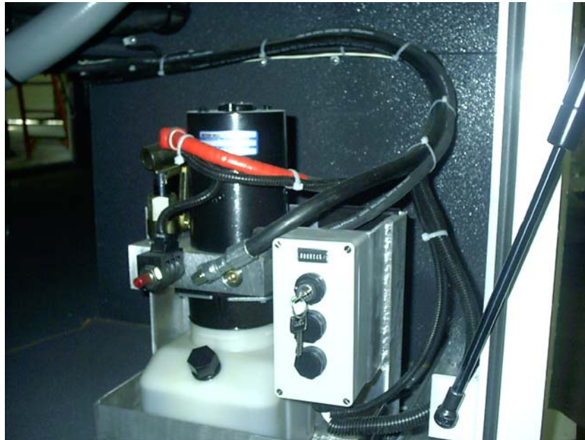
Figure 44: Platform Lift Service & Maintenance Controls
