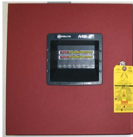
Figure 19: Fire Alarm Control Panel
