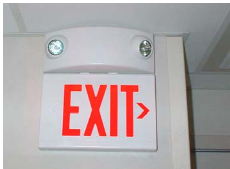
Control Room Emergency Light
