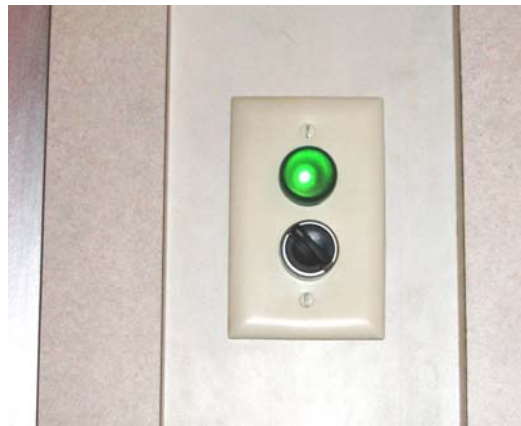
Figure 41: Platform Lift Power Switch
