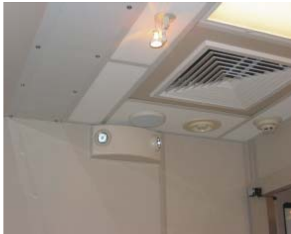
HVAC Vents Discharge
