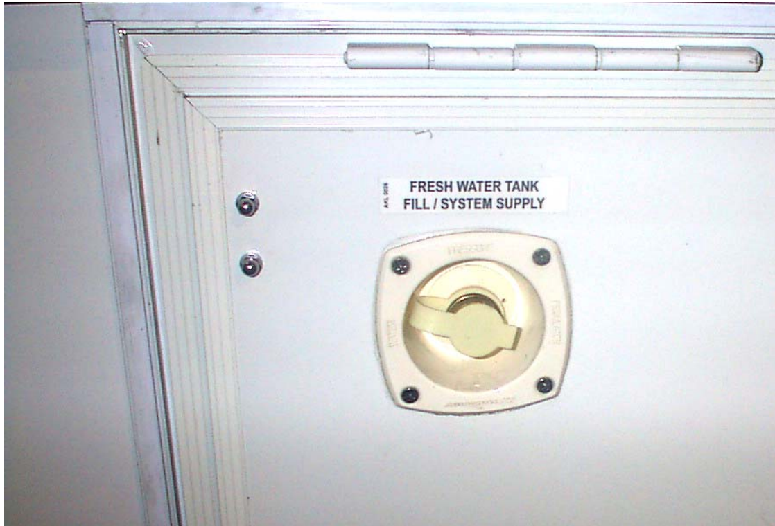
Figure 33: Fresh Water Connection
