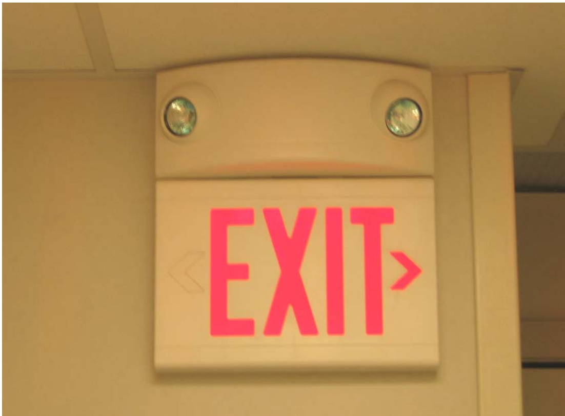
Figure 16: Control Room Emergency Lighting
