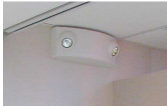
Gantry Room Emergency Light
