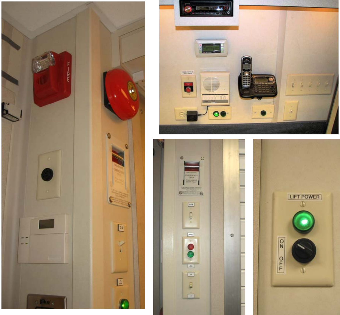
Figure 11 Mobile Unit Controls
